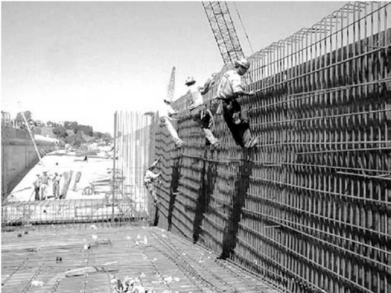
Fig. 2.2.2(b)—Stirrups to resist shear in a concrete box girder bridge (courtesy HDR Engineering, Inc.).
