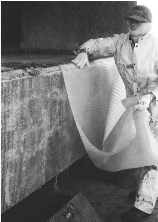
Fig. 3.4.2—Installation of FRP sheets on a reinforced concrete beam (courtesy of Hexcel Fyfe Co.).
