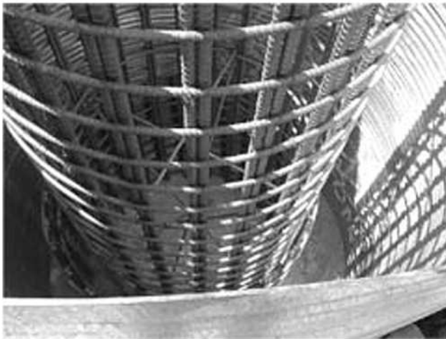
Fig. 2.2.2(c)—Hoop reinforcement in a reinforced concrete column (courtesy of HDR Engineering, Inc.).
